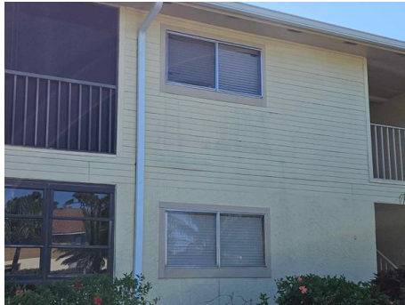
No Protection Throughout
