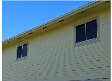
No Protection Throughout
