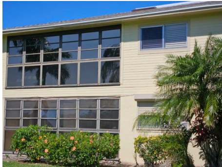
No Protection Throughout
