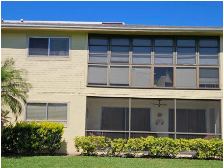
No Protection Throughout
