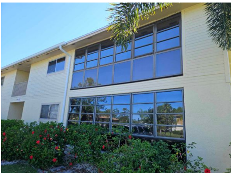
No Protection Throughout
