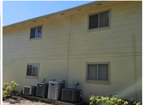
No Protection Throughout
