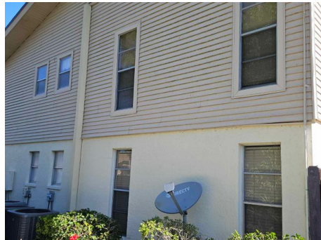
No Protection Throughout
