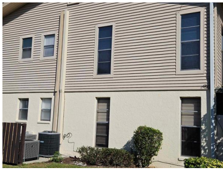
No Protection Throughout
