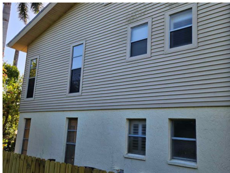
No Protection Throughout
