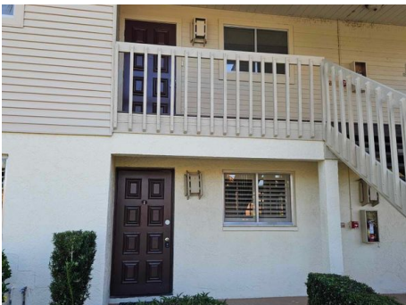
No Protection Throughout
