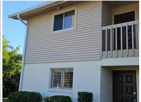
No Protection Throughout
