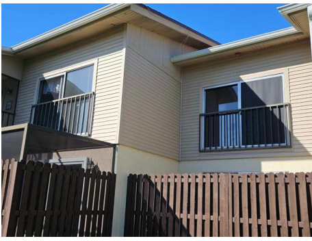
No Protection Throughout
