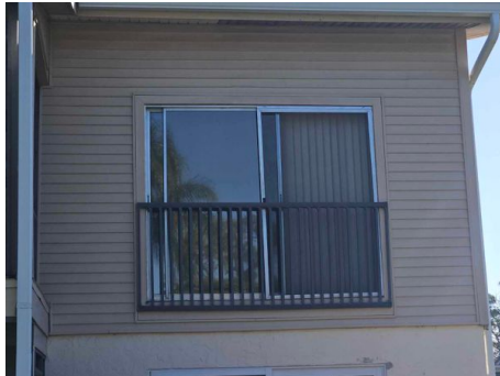
No Protection Throughout
