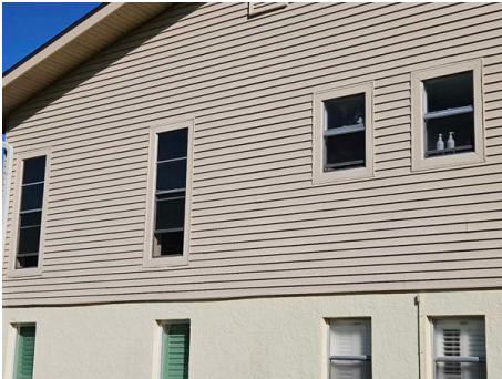
No Protection Throughout
