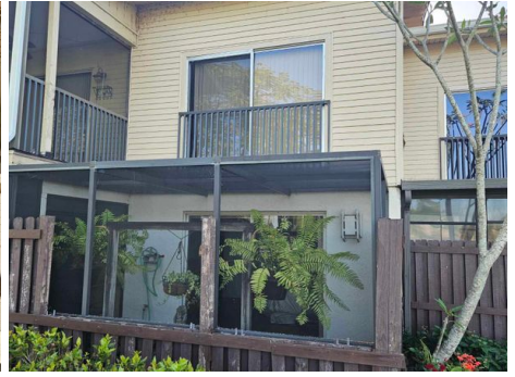
No Protection Throughout
