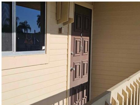
No Protection Throughout
