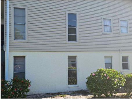
No Protection Throughout
