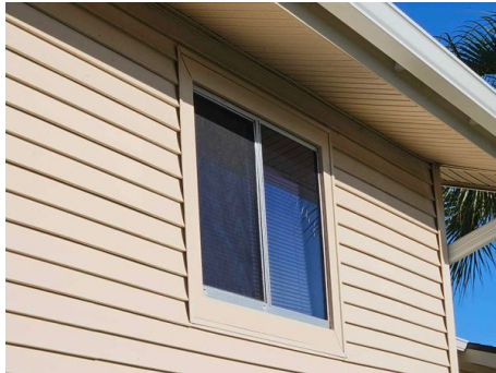
No Protection Throughout
