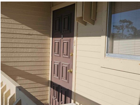
No Protection Throughout
