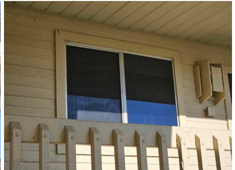
No Protection Throughout
