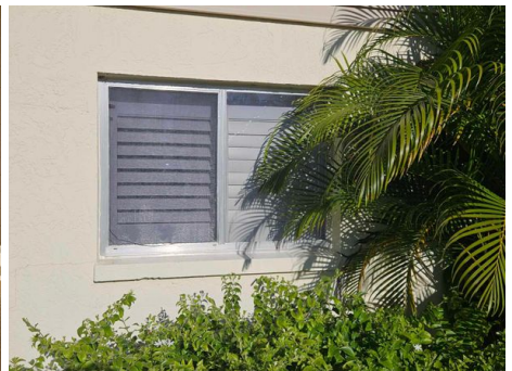
No Protection Throughout
