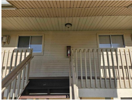
No Protection Throughout
