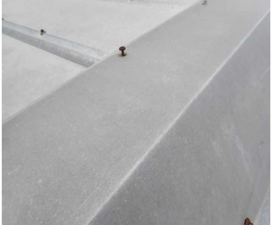
21. Deficiency #3 - Loose fasteners
