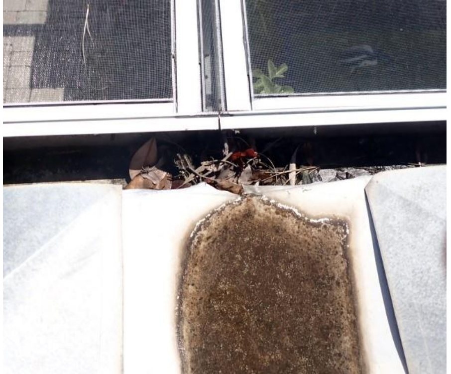
13. Deficiency #1 - Debris in gutter
