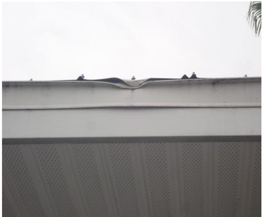
Deficiency #2 - Damaged / dented metal panels
