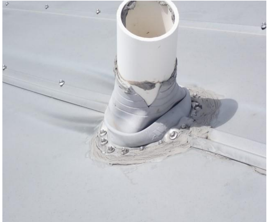
13. Deficiency #1 - Deteriorated pipe flashing detail
