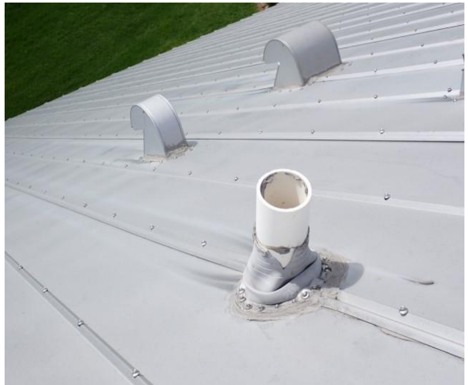
14. Deficiency #1 - Deteriorated pipe flashing detail
